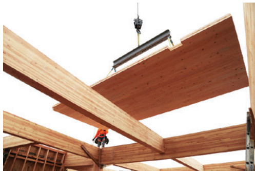
Building kits include prefabricated elements or sections that are then delivered and assembled on-site. The kit-of-parts approach, via panelization, is typical for mid-rise wood buildings. Image courtesy of LEVER Architecture
