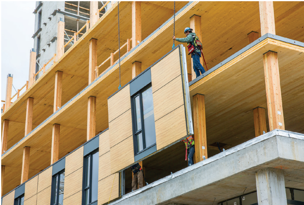
The foundation, ground floor, second-floor slab and stair/elevator cores are concrete, while the superstructure is composed of prefabricated cross-laminated timber panel floor assemblies supported on glue-laminated timber and parallel strand lumber columns with steel connections. Image courtesy of naturallywood.com
